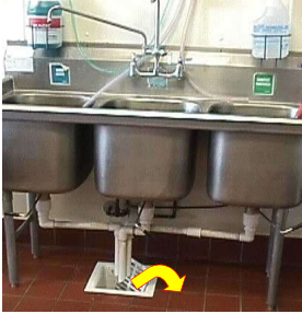
Sewage back up potential
