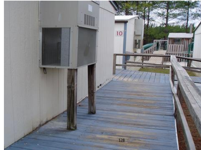
Poor condensate drainage
