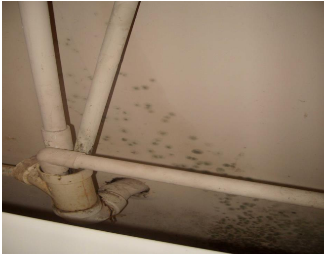
Poorly designed condensate drain
