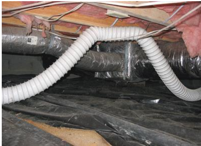
Poorly installed clothes dryer vent
